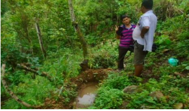
Eye-brow trench to collect and infiltrate rainwater
